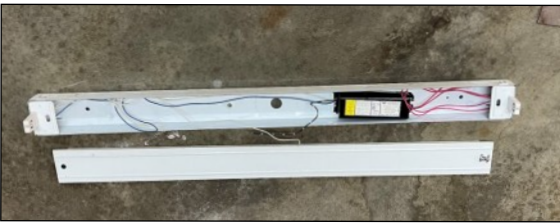
4ft florescent light fixture - -- works, no bulb
