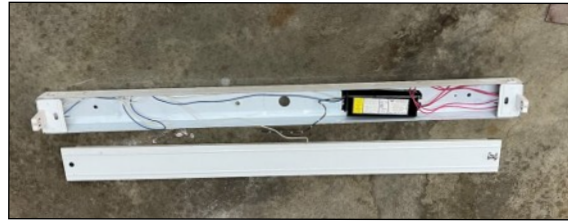
4ft florescent light fixture - -- works, no bulb
