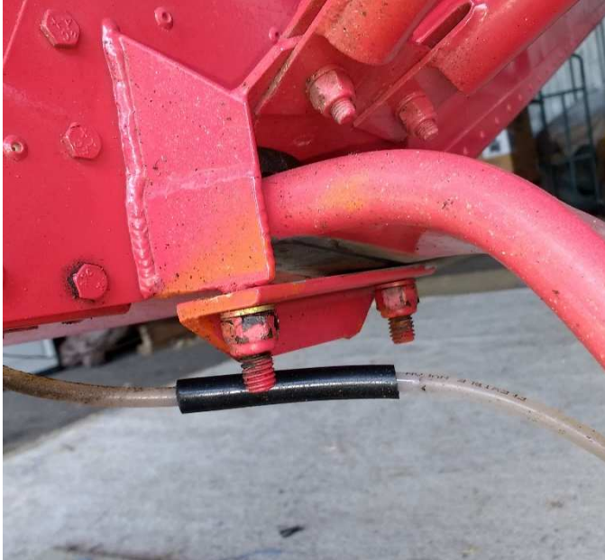
Missing clamping blocks allowing the gear to sit at an angle and rotate within the fixture
