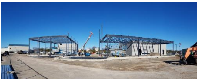
In this picture shown above is the structural steel is on its third week of being placed. This photo was taken on December 20, 2020 for the official Whitman Regional Airport's Facebook Page.
