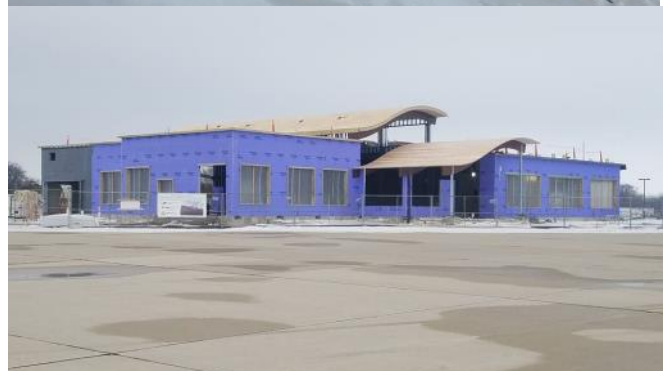
In these picture shown above: The beams are set over the lobby space and roof decking is being installed over top. Not too long now and we'll be enclosed, working inside with some temporary heat!! This photo was taken on January 6, 2021 for the official Whitman Regional Airport's Facebook Page.
