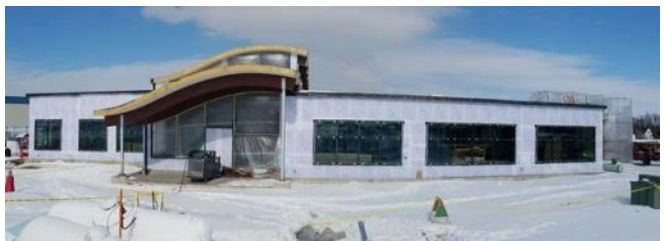
In this photo shown above: Windows are being installed and work continues at a brisk pace on the interior. This photo was taken on February 18, 2021.
