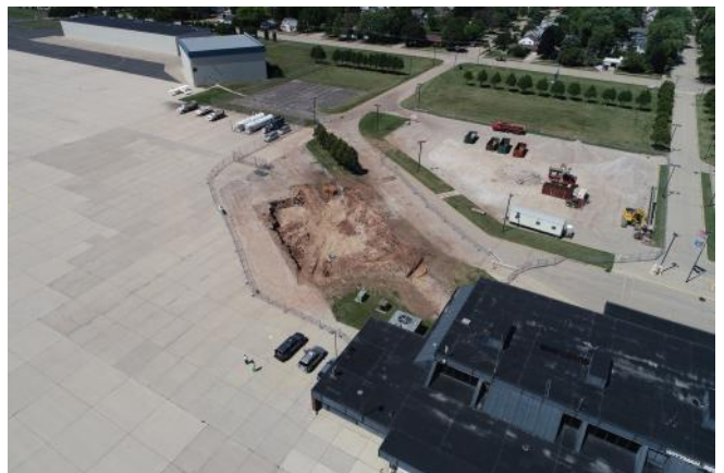
This was the site of the Basler Flight Service. They are now in the main terminal. They will be in the new terminal until the completion of the general aviation terminal.
