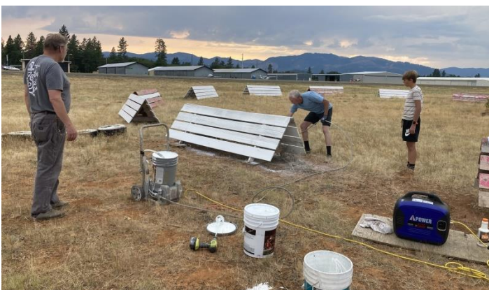
Jim gets the paint party started as Steve and Porter look on, ready to move the generator and paint cart to the next section.
