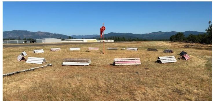
Lots of progress for just over 2 hours spent. Repaired, reset, and ready for paint.
