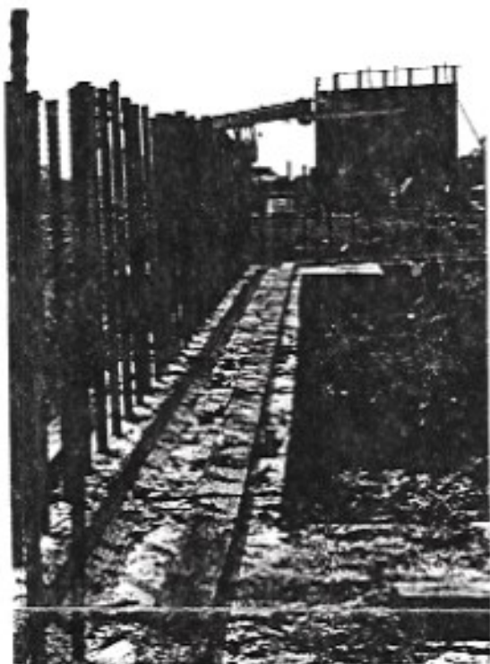
"Concrete evidence" of progress on the new EAA Aviation Center being constructed at Oshkosh. This photo, taken July 10, shows footings and "re-bar" in the office area with a wall of the reception area rising in the background.
