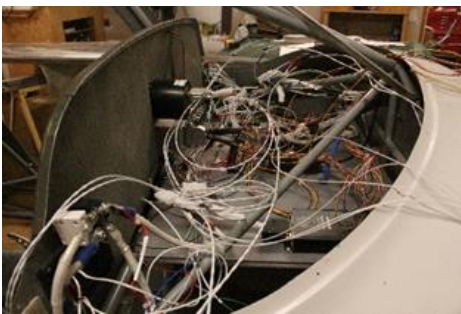
WIRES EVERY WHERE
