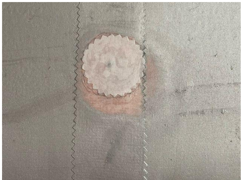
The “dollar patch” repair glued over the puncture with POLY TAK adhesive.
