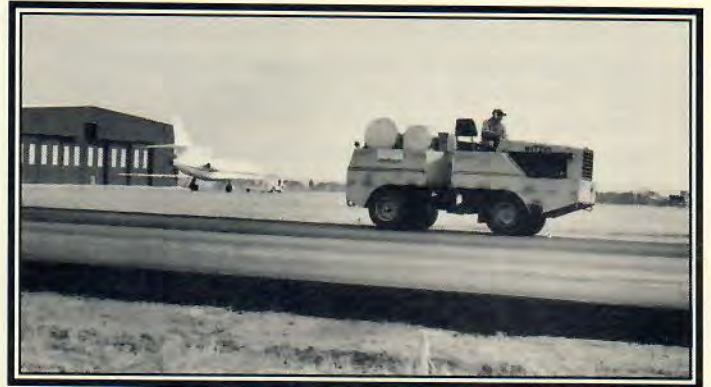
Pavers work to lay asphalt for new taxiway at Jeffco Airport. The taxiway will improve traffic flow in a heavily traveled area.
