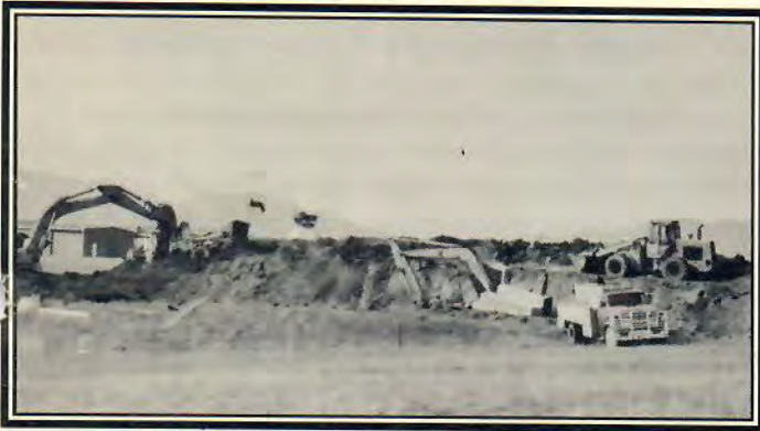
Construction crews work on trenches to house 2500 feet of sanitary sewer lines at Jeffco Airport.
