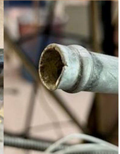
Photo 3: Mud in plumbing.
