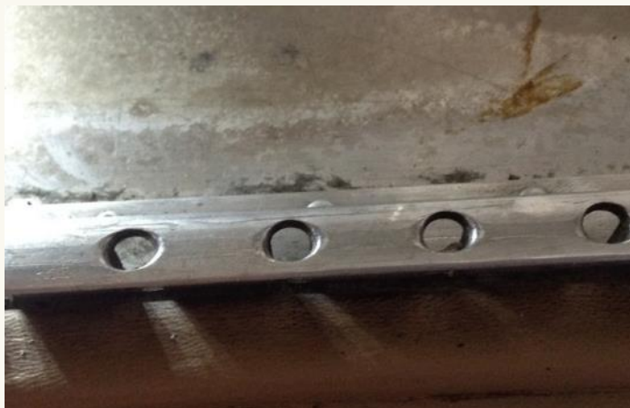
Photo 1: Cessna seat rail with rounded holes. These holes are still in limits, but not by much.
