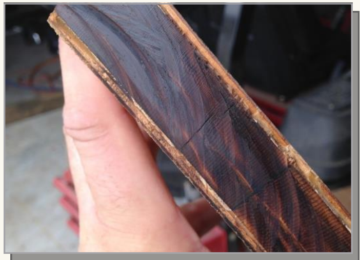
Photo 3: Upon removing the spar - vertical cracks under the plywood doubler. Photo Credit, Doc Hecker
