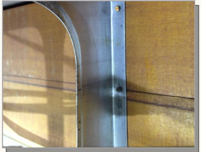
Photo 2: Large horizontal cracks. You can catch a finger-nail in these! Photo Credit, Doc Hecker
