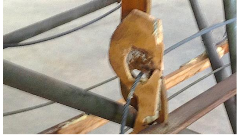
Photo 4: There is a proper way to make a scab patch on a wooden structure, but this is not it.
