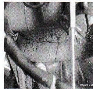
Figure 3. Melted Oil Temp Insulation
