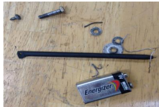
Photo 2: Items found at the tail post during a recent inspection
