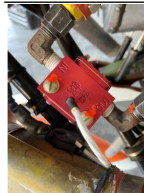
Photo 5: Fuel flow transducer
