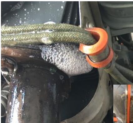
Photo 5: Bubbles at an exhaust flange.
