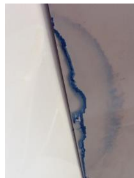
Photo 10: Same place, fresh fuel stain. This is a running leak – dangerous.
