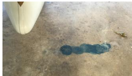
Photo 8: Fuel stain on the floor. This should get your attention!
