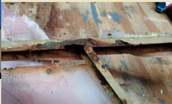
Photo 3: The bottom rudder rib (horizontal piece) is rusted away from support structure. The fabric was bulging over the rust blister.
