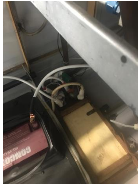
Photo 4: New location of solenoids and breakers on a Decathlon. The battery is waiting to be placed on the plywood platform. This is located behind the baggage bulkhead panel.
