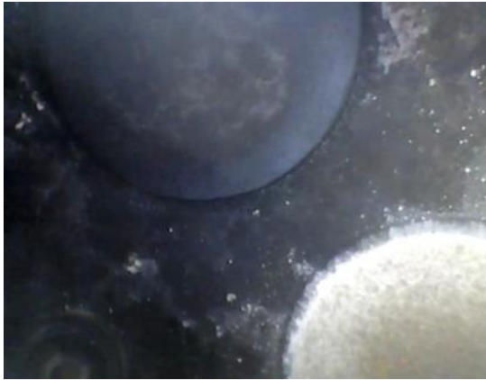
Photo 3: Borecope of the valves inside a fairly clean cylinder.
