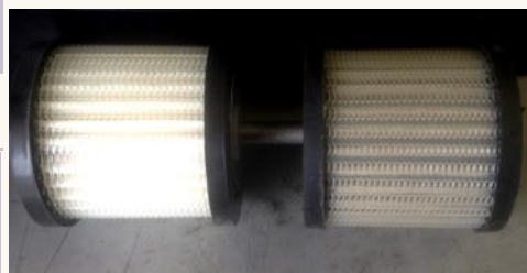
Central Vacuum Filters, New and Way Past Due
