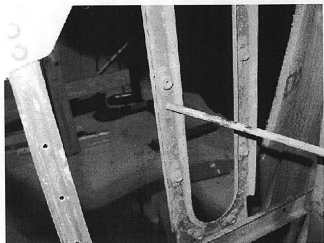
Figure 4 - Surface corrosion around pushrod control cut-out. Note deteriorated fiber locknut plates and improper drilling of rib flanges for fabric support by pop-rivets instead of rib stitching.
