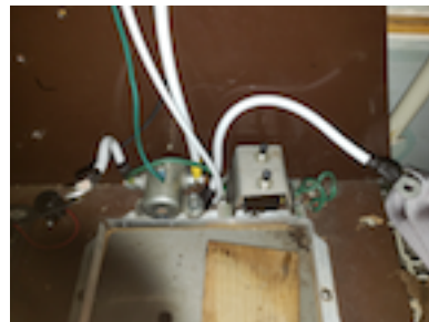
Mark's new battery box . . .
