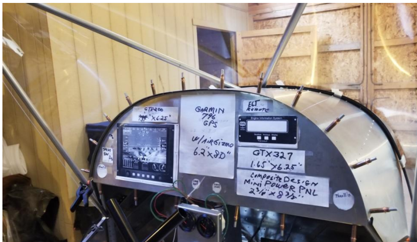
Blind side look of Cleco Fastener holding curved aluminum dash to faceplate.
