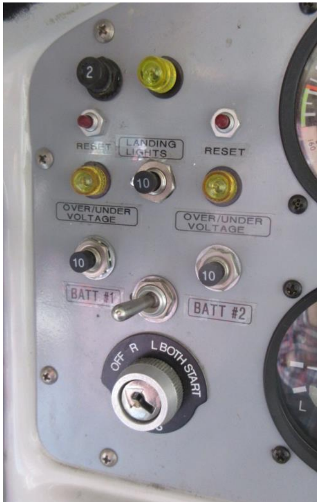
Part of the panel when I bought the plane. It had two electrical systems and some mysterious, unlabeled circuit breakers.
