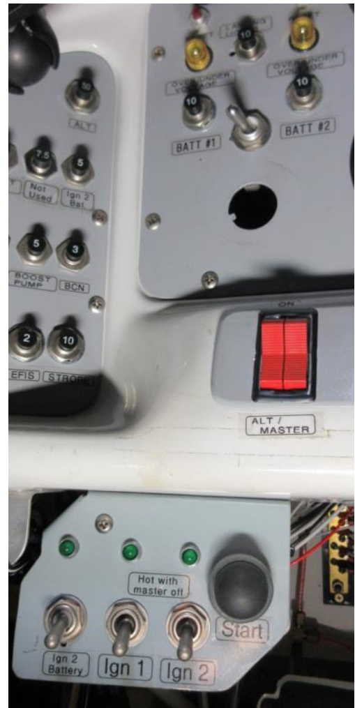
The first set of changes included removing the key start switch and adding a temporary panel with separate ignition system switches.
