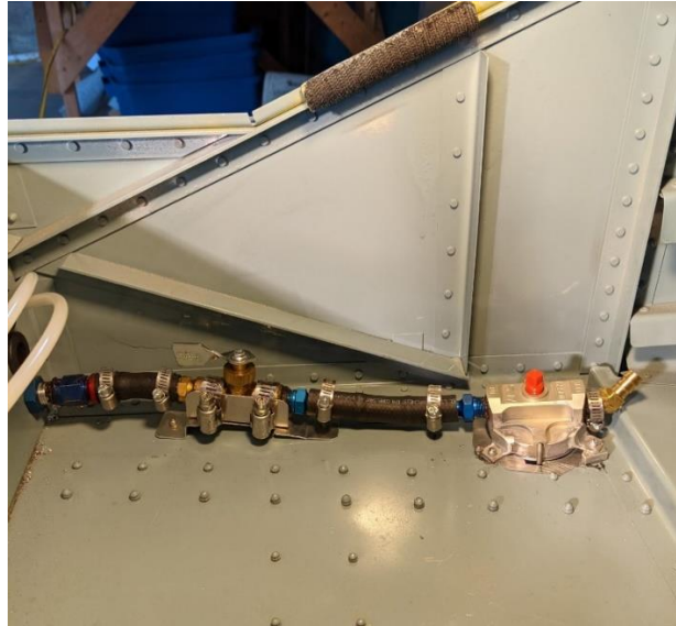
Figure 2. Fuel line at the pilot side and below the door sill with the shutoff valve and gascolator in place. A protective sheet metal cover will eventually be fabricated to cover this assembly.
