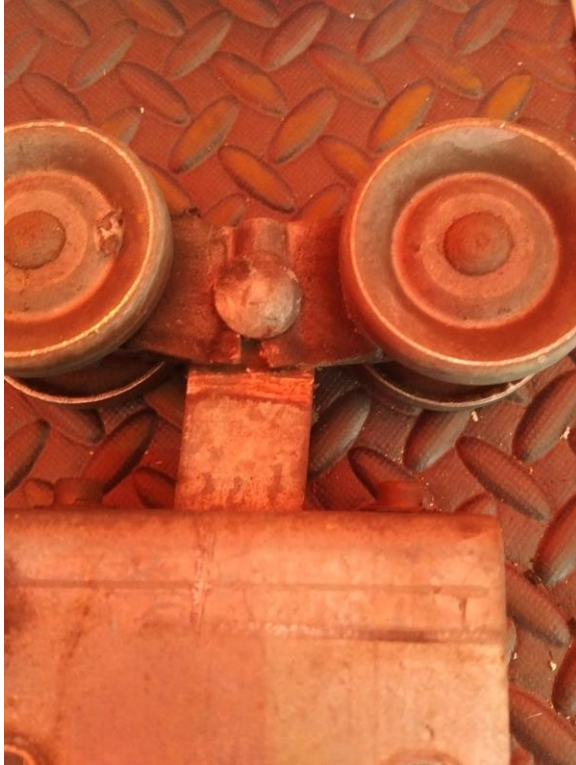
Photo five: Cracking sagging Hanger bracket
