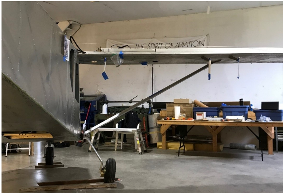
Figure 3. The starboard strut has been cut to final length and bolted in place at the top and bottom mounts. The port strut was installed in the same manner and the wings now became self supporting.
