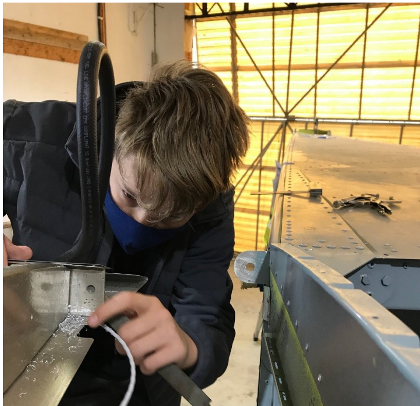
Figure 1. Our youngest builder, Colin, is busy deburring the newly drilled bolt hole in the rear spar for the rear wing mount bolt. The hole was drilled up to size then a finish size reamer was used, the matching hole can be seen in the grey tab protruding from the fuselage side.
