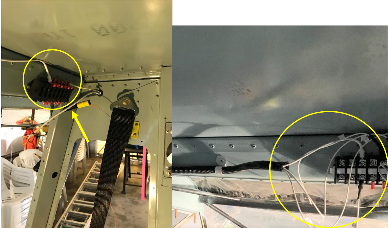
Figure 2. Terminal block installation (circles) on the rear side of the mid-cockpit upper cross member on the copilot/passenger side. The black conduit (yellow arrow) will take the common wires down and forward to the instrument panel.
