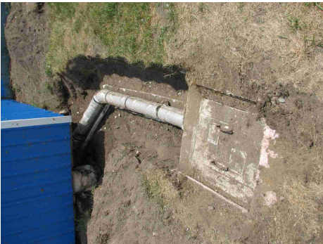
There is still work to be done on winterizing the septic system
