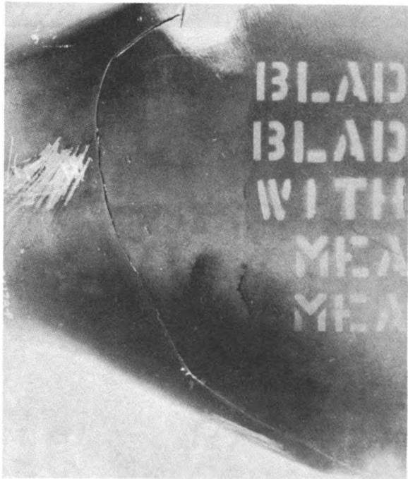
Figure 4.47.—Rib termination fillet failure.
