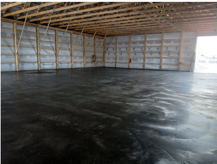
Here is what a nice finished cement pour looks like for Scott's new hanger.
