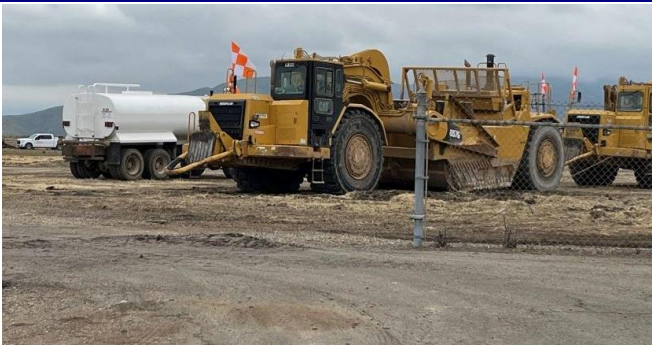
San Diego MetroPark construction finally under way. Big equipment and security fencing are affecting access to the Chapter leasehold. Old Charlie is permanently closed, but access past the Tower remains as normal. 4/23
