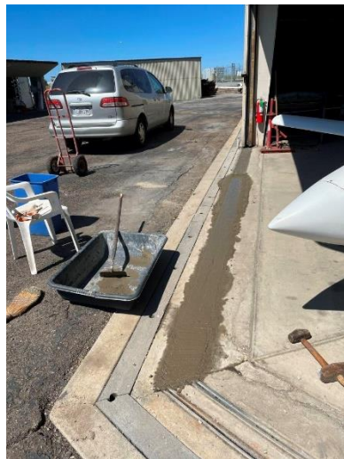
Concrete maintenance on the SW corner of Hangar 3. Thanks to Nigel Worrall and Ryan for taking this on. 3/23
