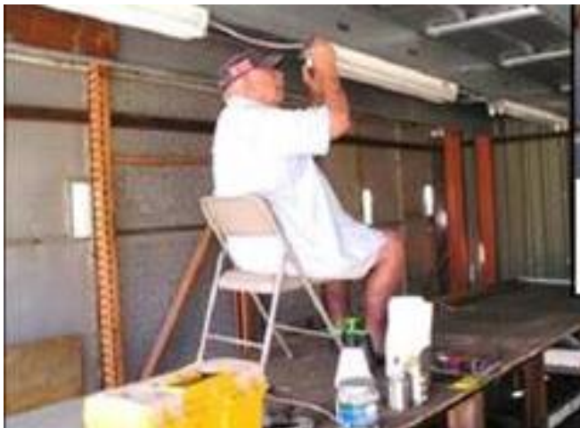
Sitting down on the job. Jimmy Kennedy installs lighting in the new Playboy (#8) hangar in 2014. The story goes that much of the hangar structure is re-purposed Home Depot lumber shelving.
