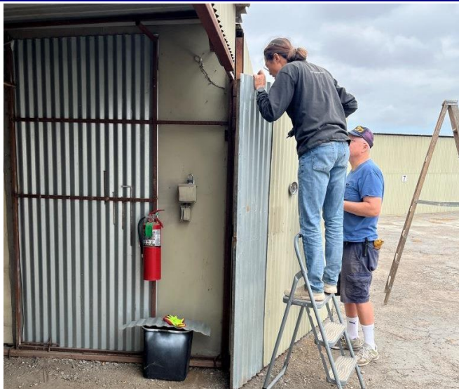
Adam L. & Mike B., with help from Ryan, make repairs to a hangar door on October 17 th . We depend on help from our volunteers to keep our Chapter functioning.
