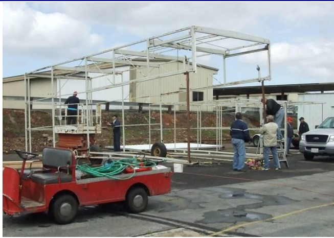
Disassembly at MYF—the first stage of moving a hangar donated by Buzz Gibbs.
