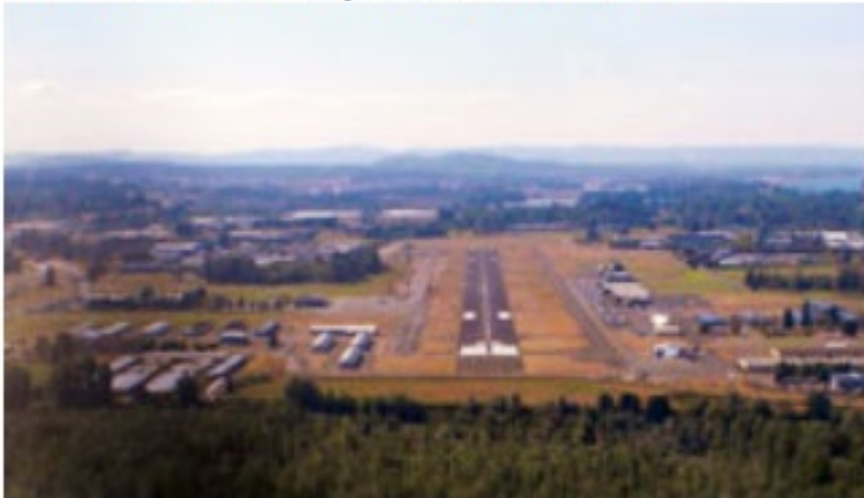
Photo taken 03-Sep-2008 on a 1/2 mile final for runway 25, shows taxiway B expansion and widening in progress
