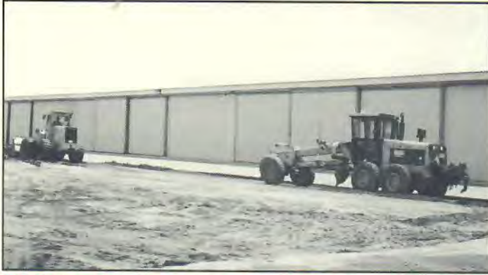
The T-Hangar ramp areas are currently being reconstructed with the support of Jefferson County.
