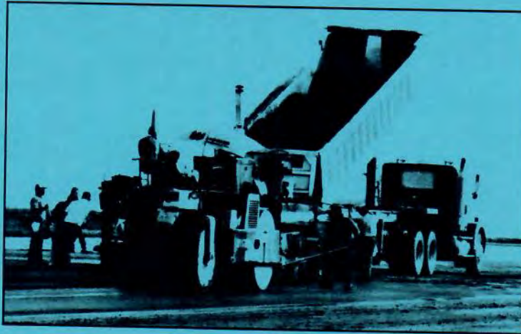
Construction crews began working on repaving the north ramp area in early June.
